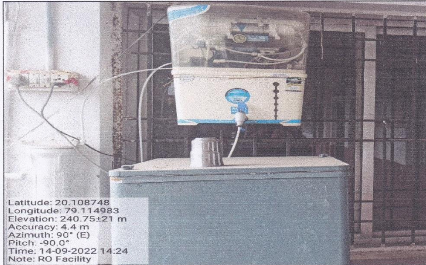
RO Water System
